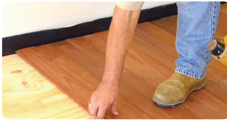
Figure 4.18: Secret fixing to a plywood sub-floor. A polyethylene moisture barrier has been placed over the slab and both the plywood and flooring are clear of the wall.
