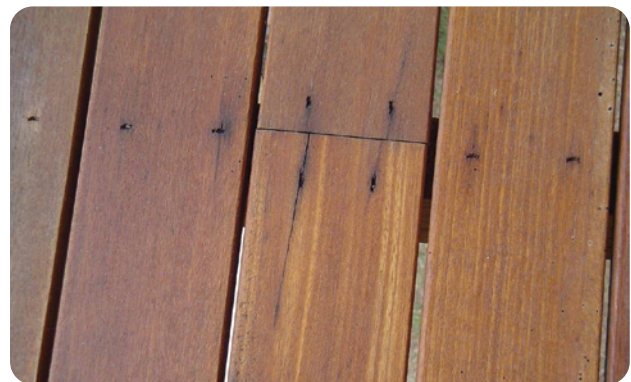
Incorrect use of non-galvanised ‘T’ head nails in decking.
