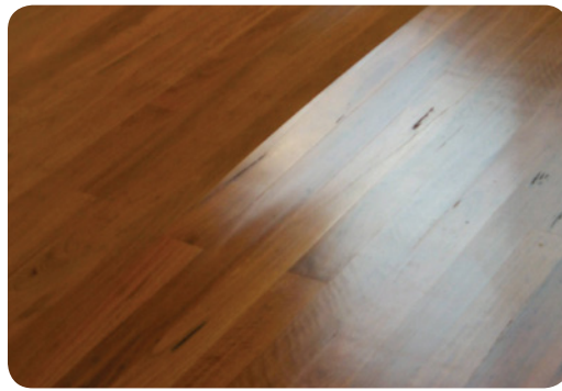
Figure G1: Tenting resulting from atmospheric moisture uptake.
