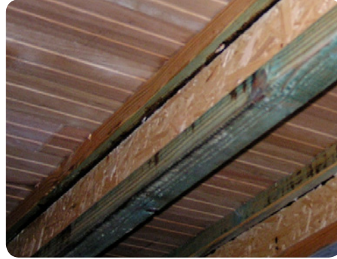
Figure 4.7: Timber floors are successfully laid over a range of solid timber and engineered joist systems.
