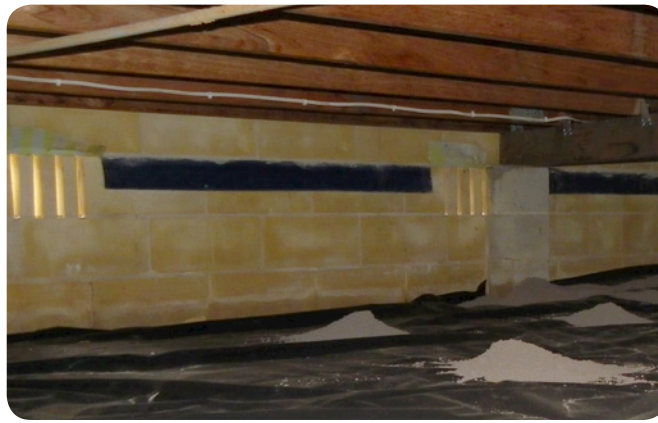
Figure 3.20: For frequently damp soil conditions, the sub-floor ground level can be raised with crusher dust and a polyethylene membrane laid over it.
