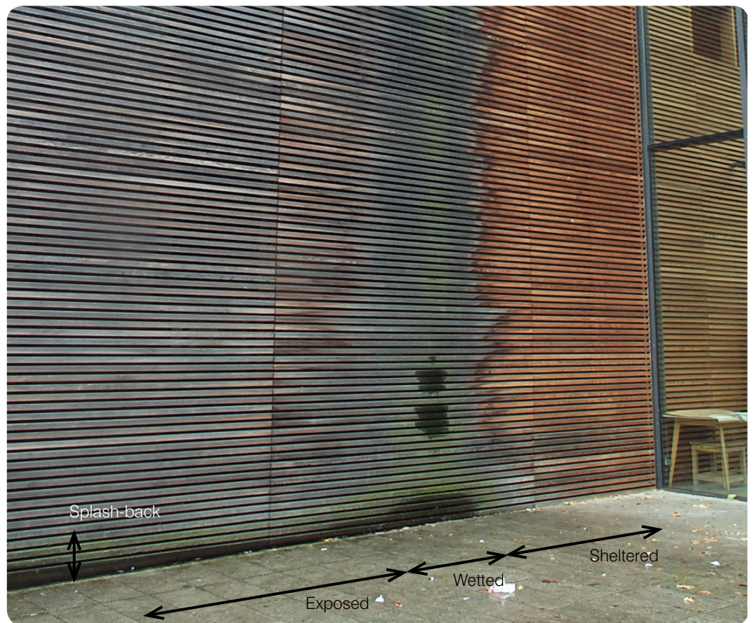
Figure 6: Differential weathering and decay on a facade.
