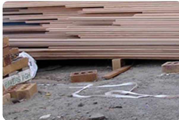
Figure 3.1: Inappropriate site storage can void manufacturer warranties.
