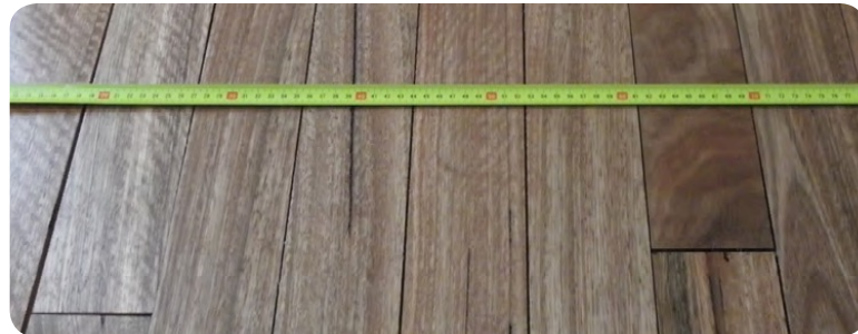
Figure 9.7: Gapping that is not considered acceptable.
