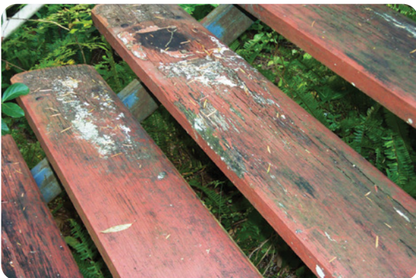
Poor maintenance of stair tread.
