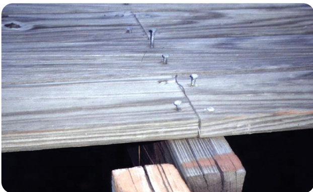
Plain shank decking nails in pine have ‘worked out’ with cyclic wetting and drying.
