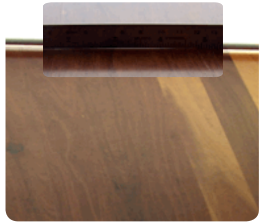
Figure 9.4: Cupping – Board edges higher than the centre of the board, but which is barely visible in the floor.
