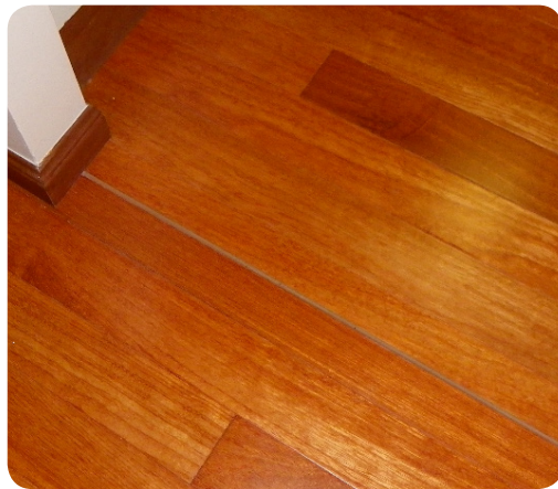
Figure 7.5: Caulked joint used to relieve potential expansion pressure through a narrower doorway linking two larger floor areas.
