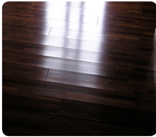
Figure 7.3: Peaking due to expansion pressure.
