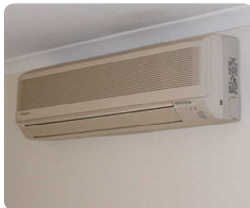
Figure 3.13: In warm climates these units are referred to as reverse cycle split system refrigerative air conditioners. In cold climates such as New Zealand they are referred to as heat pumps.
