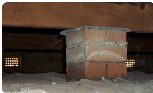
Figure 3.15: A dry sub-floor space and adequate ventilation is essential for floor performance.
