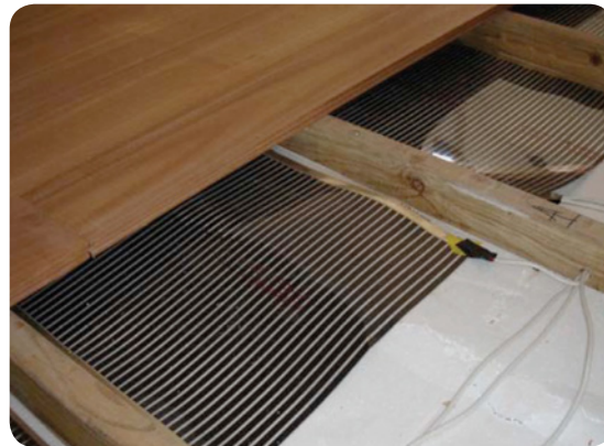
Figure E3: Blackbutt flooring (130 mm wide) with electric underfloor heating in Adelaide.
