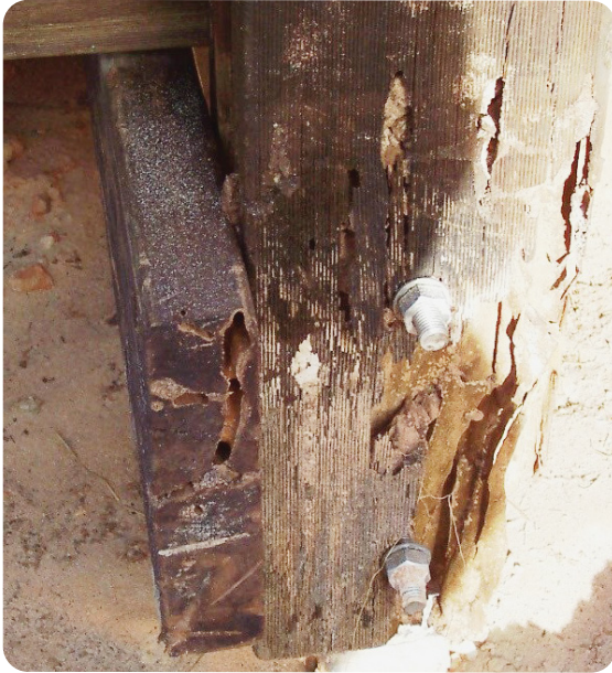
Termite damage to non-resistant timber.
