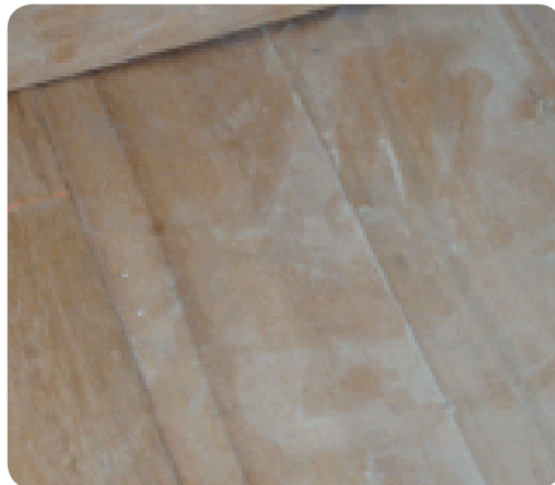
Figure 8.1: Prior to sanding, the floor should be assessed to ensure that it is in a condition suitable for sanding.
