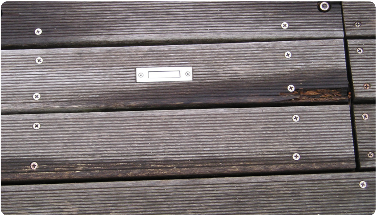
Decay in untreated sapwood on edges of decking boards.
