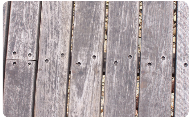
No splitting of joists where deck screws were staggered.
