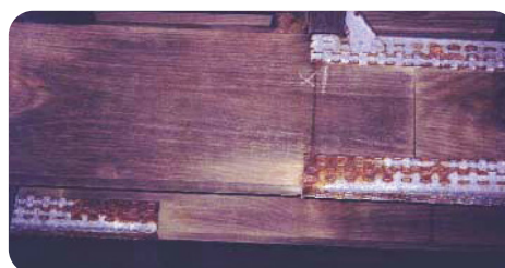
Corrosion of nail plates on deck joists after 6 years exposure near surf beach.
