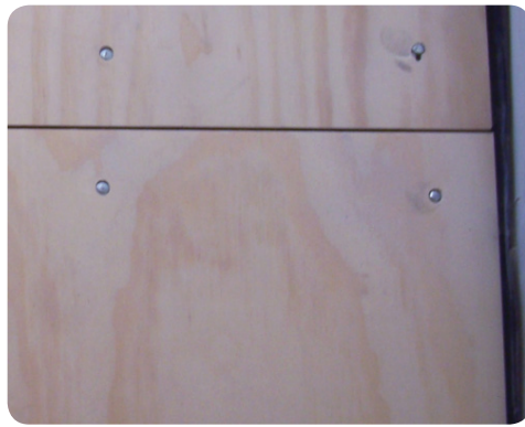
Figure 4.19: Fixing of the plywood sub-floor through the polyethylene membrane and into the slab.
