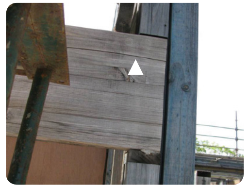
Split (indicated by arrow) along second top laminate (does not follow glue line) at end of beam.
