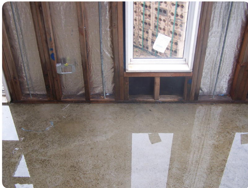
Water ponding on slab. Note wicking of moisture up the studs.
