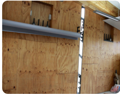
(b) Wall anchorages and UFPs with no fire protection. NMIT building.
