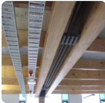
(a) Exposed tendons, no fire resistance.
