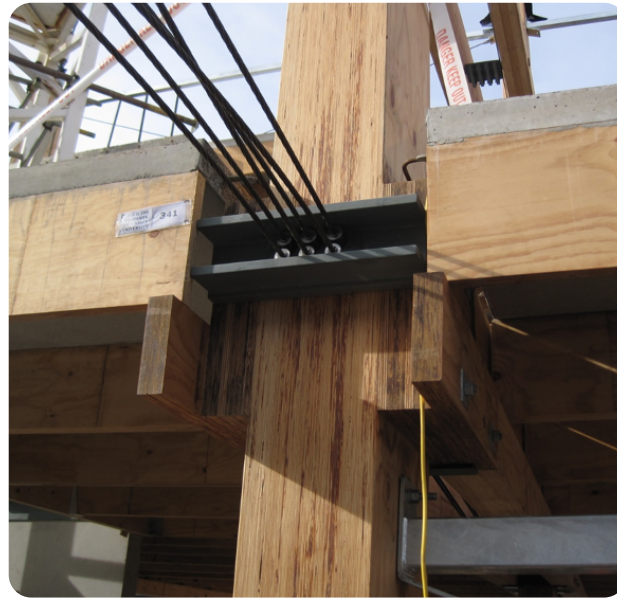
Figure 4.1: Post tension Frame Massey University, Wellington, New Zealand. (Image credit: STIC)
