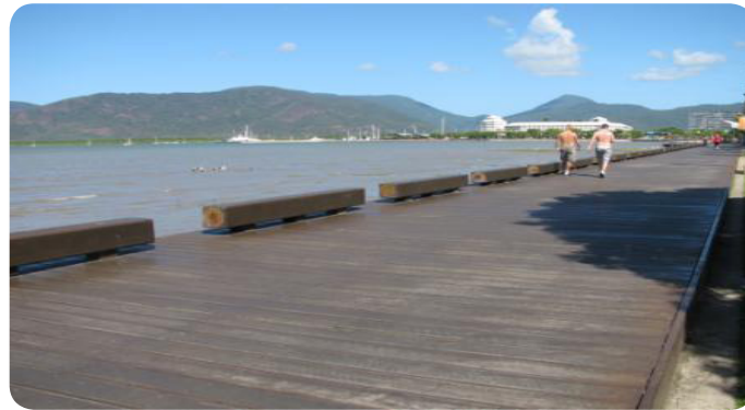
Figure 18: Site-applied pigmented deck stain requiring maintenance.
