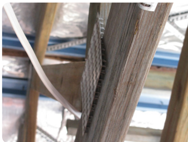
Loose truss plates where trusses exposed to weather for six months (prior to roofing being installed).
