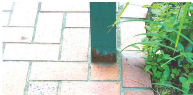
Significant corrosion of embedded galvanised steel post bracket.
