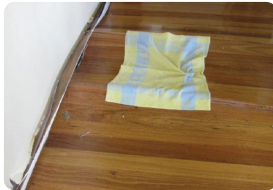
Tenting of T&G floor due to prolonged moisture being trapped under the floor. This inundated T&G floor supported on a particleboard sub-floor 'tenting' about one week after the flood water receded.
