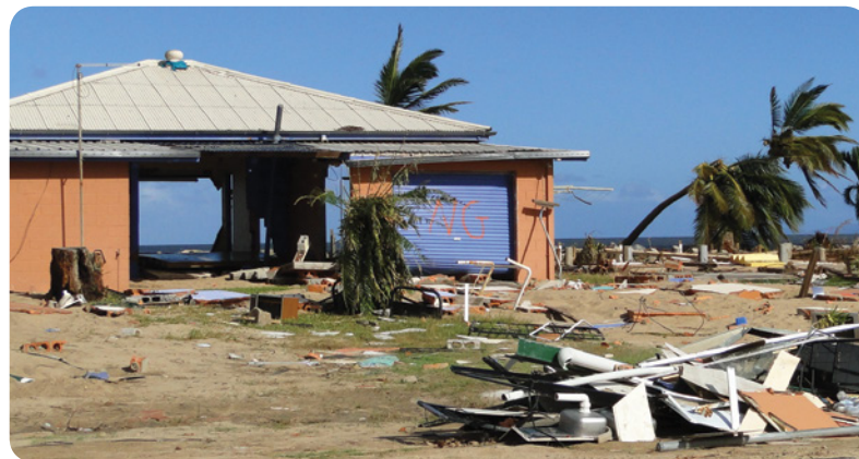
Storm surge damage to a slab on ground house. (Image: Cyclone Testing Station, James Cook University, Townsville)
