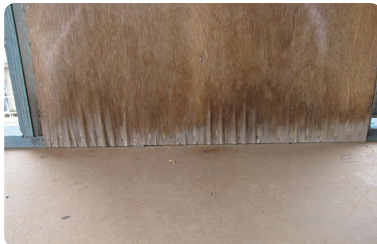
Plywood delamination at bottom plate in bracing panel. Note: The plywood used in the construction in the above example had no identification stamps or indication of certification schemes or Australian Standard for its manufacture.
