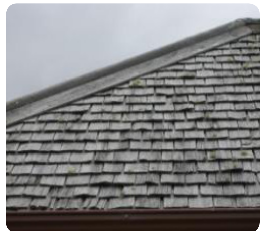
Figure 12: Bare timber shingles.
