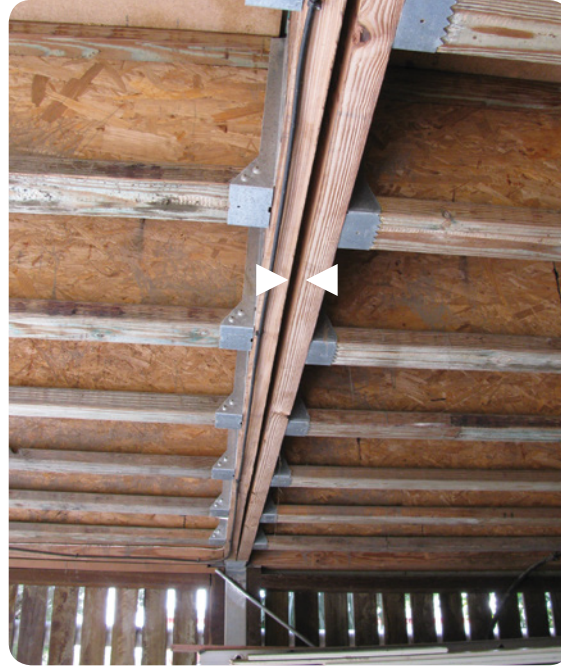
Expansion in flood-affected timber flooring.
