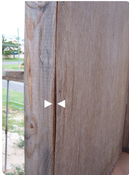
Delamination of plywood sheet bracing (see arrows).
