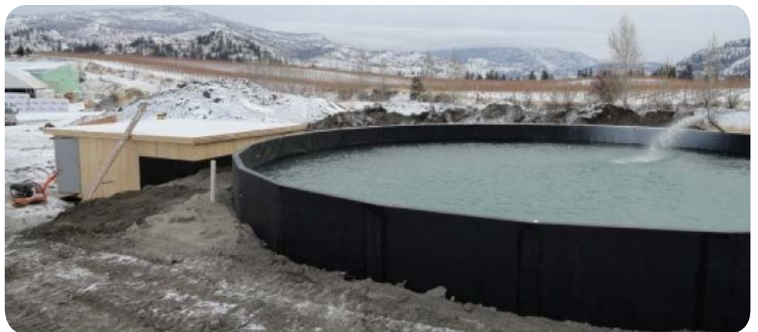
Figure 1.5: Water reservoir. Photograph: Structurlam
