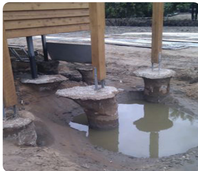
Footings scoured out by floodwaters (Image: BSA Queensland).
