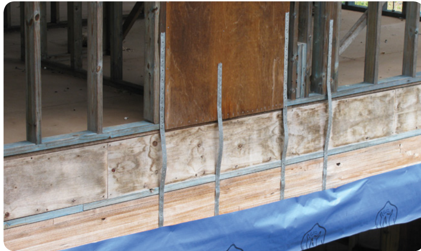
Loose tie-down steps due to timber expansion and then subsequent shrinkage.
