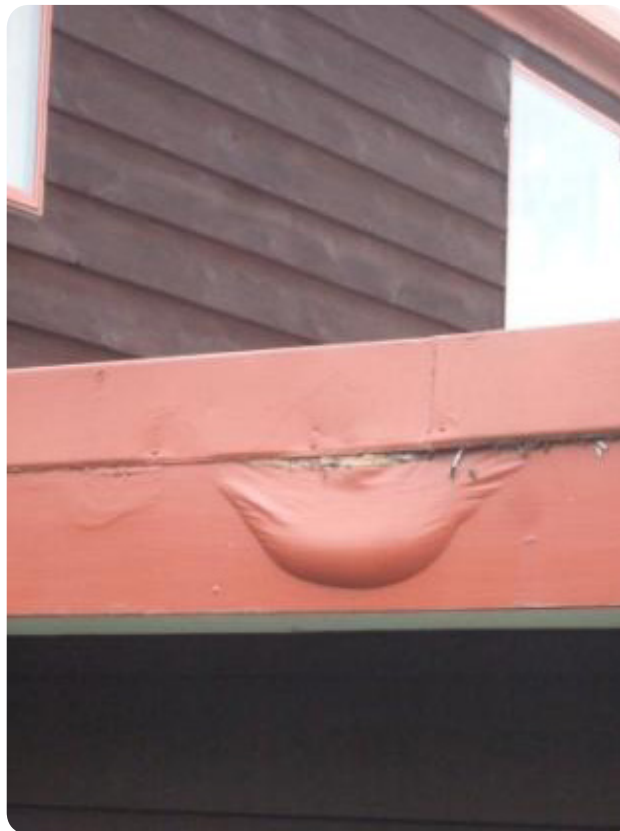
Figure 16: Poorly maintained paint which is trapping moisture.
