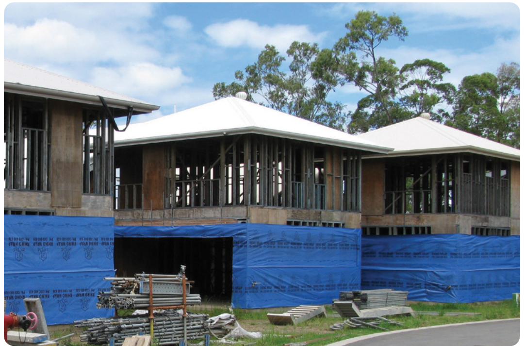
Exposed timber can become discolored and stained.
