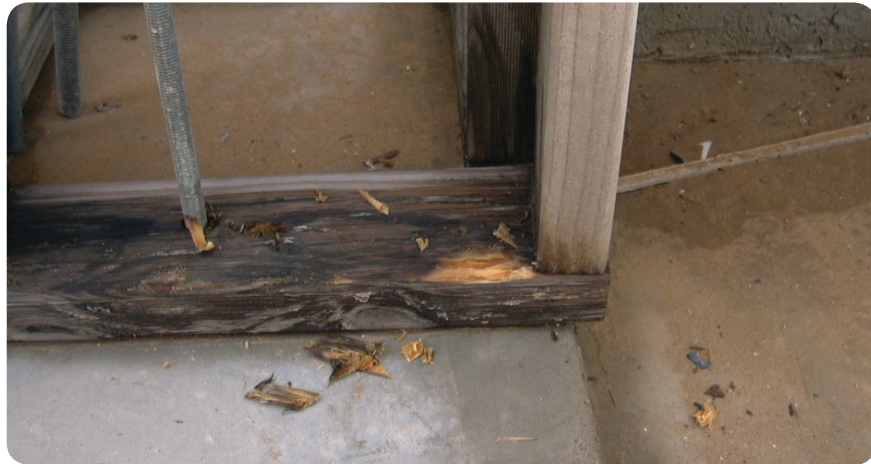
Significant discolouration due to stain but timber under surface is unaffected, with no decay.
