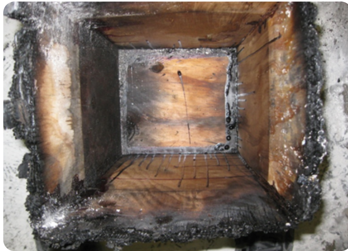
Figure 4.3: Inside a cavity carrying post-tensioning rods, post-fire. 6
