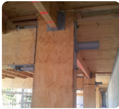
(a) Anchorages, corbels and dissipaters with no fire protection. Merritt building.
