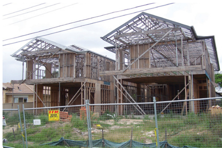
Timber frames exposed to the weather for six months.
