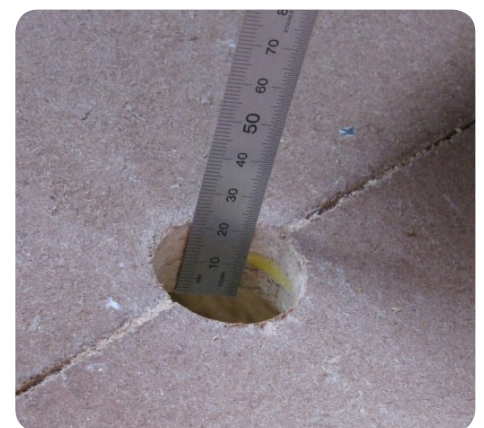
Measuring the thickness of particleboard flooring at a hole saw sample location.
