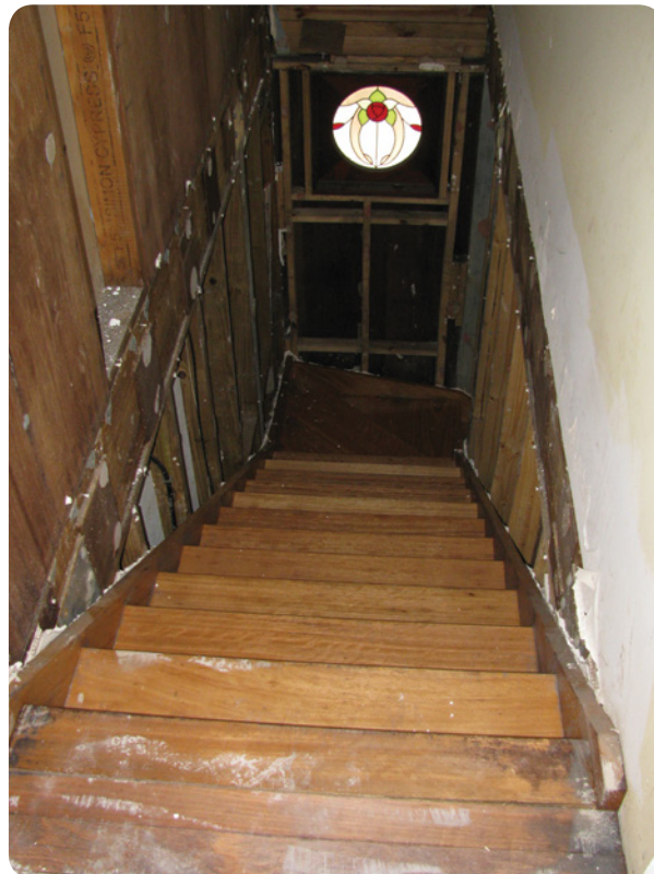
Solid timber stairs stripped out and allowed to dry were recovered following inundation.
