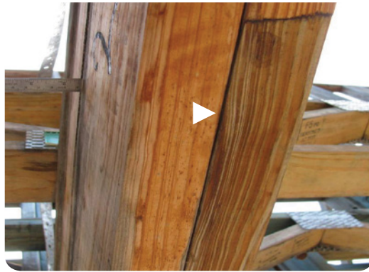
Split (indicated by arrow) totally through one of the doubled glued-laminated beams. Depth of split indicated by ruler 35 mm plus.
