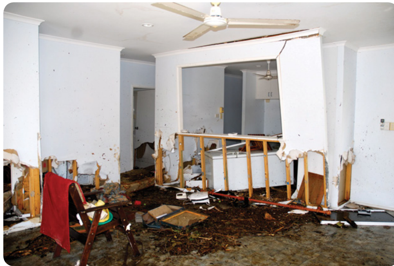
Storm surge structural damage. (Image: Cyclone Testing Station, James Cook University, Townsville)
