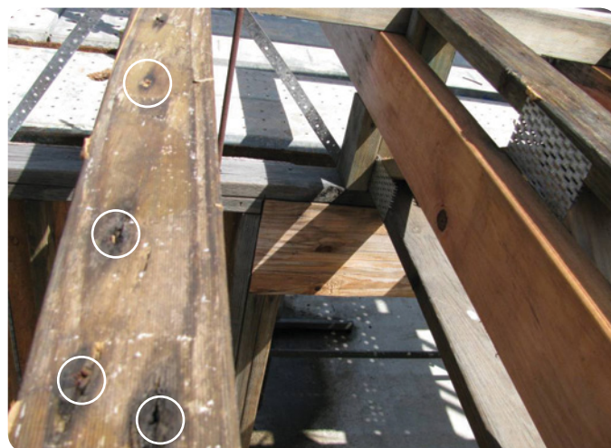
Decay pockets (highlighted) around fixing points where sheet flooring has been removed after 12 months' weather exposure.
