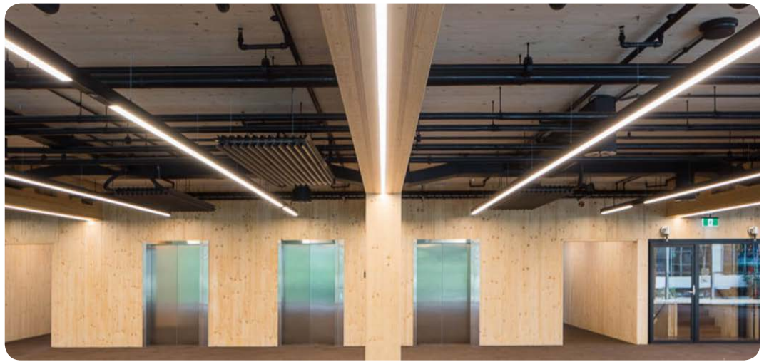
Figure 5.9: Figure 4.8: Lift installed in CLT shaft in International House, Sydney. Photograph: Lendlease
