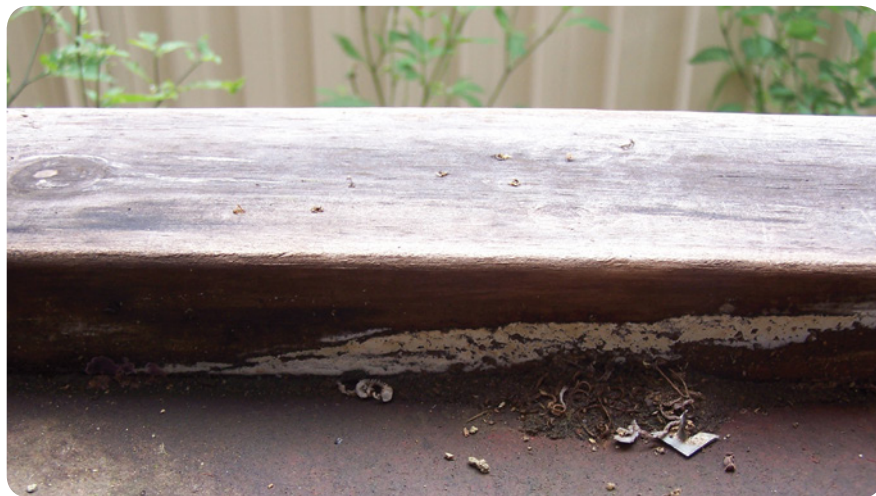
Decay in bottom plate on particleboard floor. Note small drill holes on top of plate used to detect decay.
