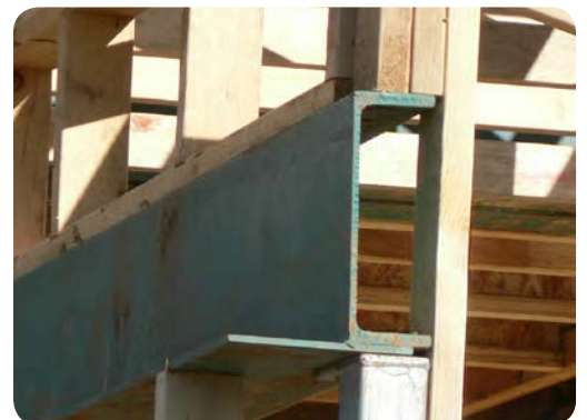
Figure 46: Thermal bridging. Beware high conducting elements that breach wall insulation. Photo: Mark Dewsbury
