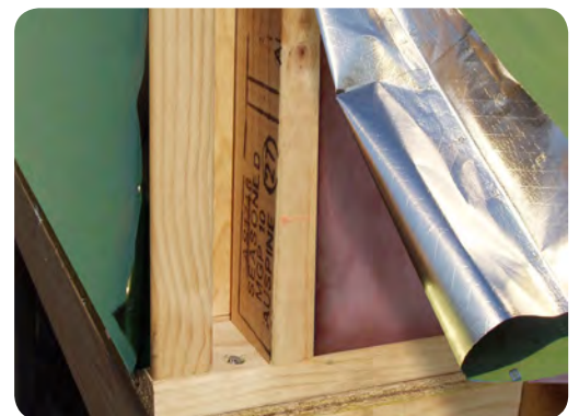
Figure 39: Lack of insulation in corners. Photo: Mark Dewsbury
