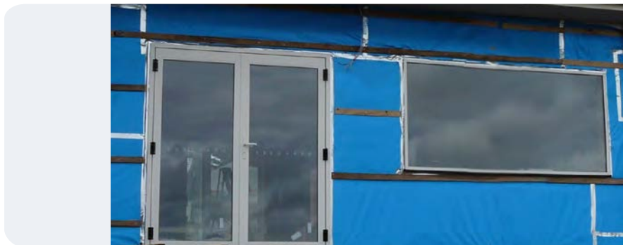
Figure 21: Tape joints. Building wrap covers all walls and is overlapped and taped. Photo: Mark Dewsbury
