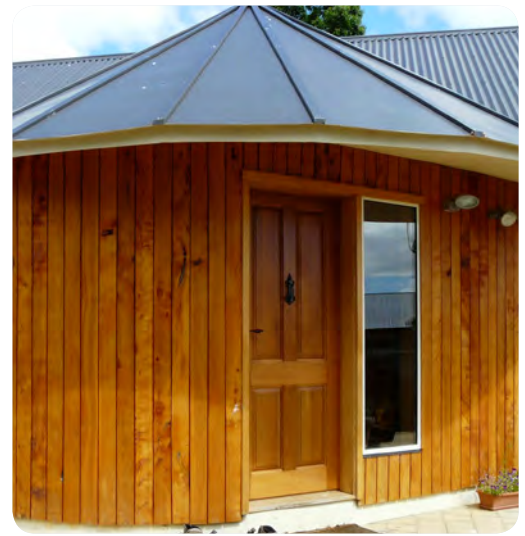
Figure 54: Traditional cladding over rigid board insulation. Timber ship-lapped boards over polystyrene board. Photo: Mark Dewsbury
