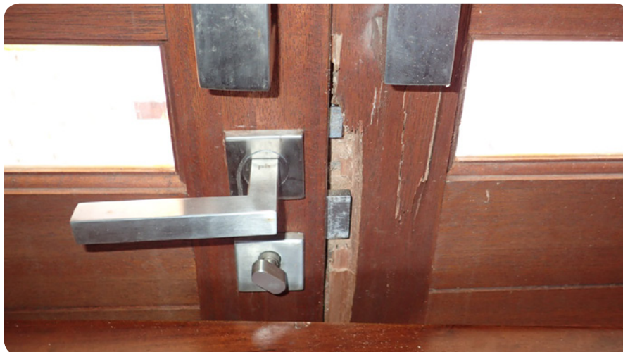
(b) Door latch failure on double entrance doors
