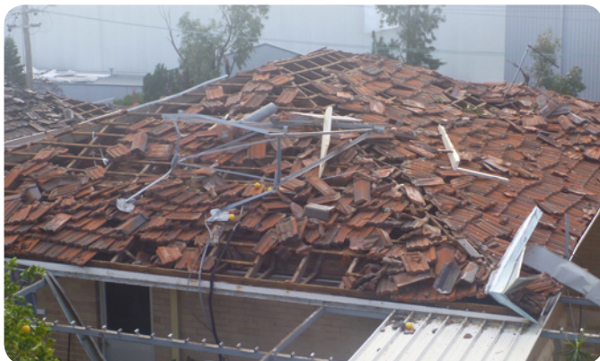
(a) Loss of tiles in Wind Region A (non-cyclonic)
