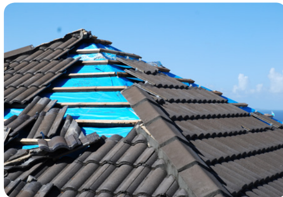
(b) Loss of tiles in Wind Region C (cyclonic)
