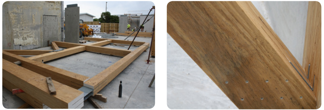
Figure 5.2: Iron stain on LVL members in wet conditions on site. (Image courtesy of Nelson Pine Ltd)
