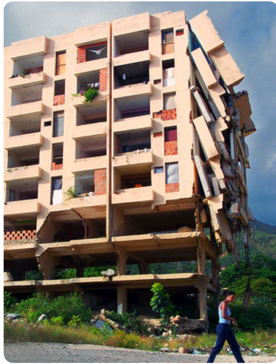
Figure 3.3: Disproportionate collapse of an apartment block in Venezuela following landslides.
