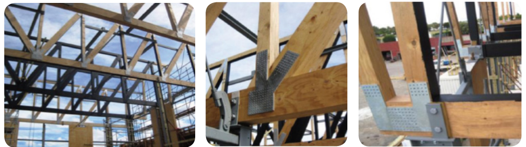
Figure 1.4: Riveted connections on the Carterton Event Centre, New Zealand. (Image credit: McIntosh Timber Laminates Ltd)
