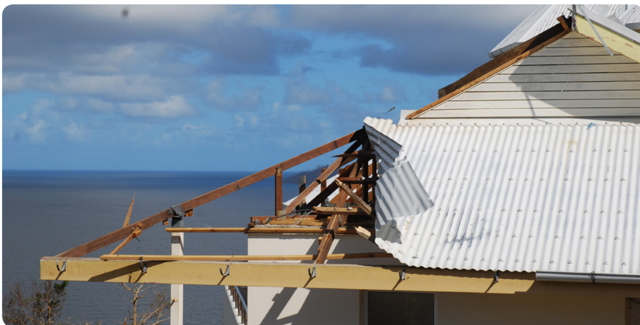
Figure 1.1: Wind damage to houses.
