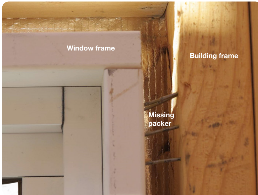
(a) Window frame separation from the building frame
