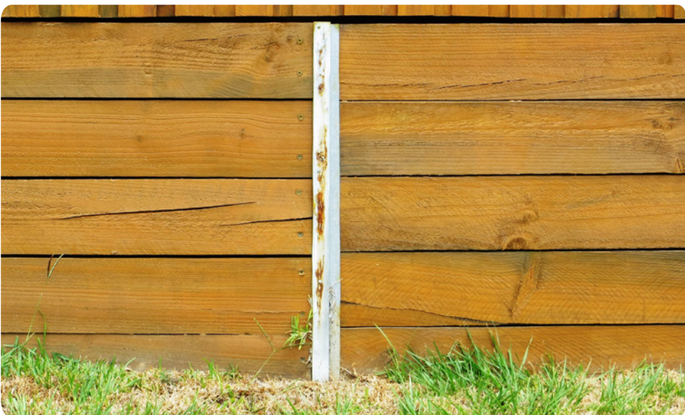
Figure 2.5: Poor quality galvanized steel 'H' section post showing corrosion approximately 8 years after installation
