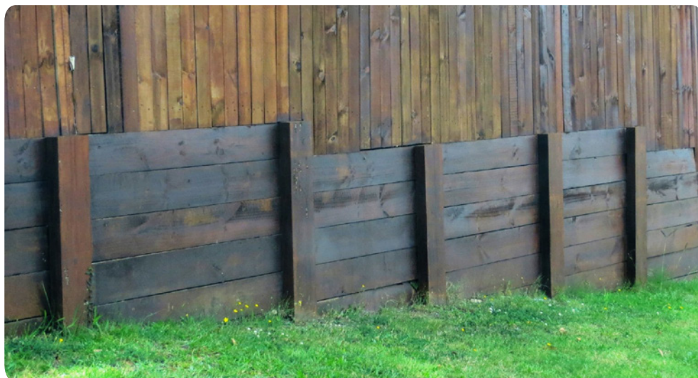
Figure 4.1: Treated pine retaining wall (and fence) being regularly maintained with application of timber preservative oil.
