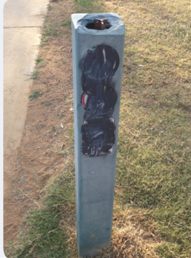
B: Reinstated – The damaged bollard is about 10 years old and is shown reinstated with the aid of a steel picket.
