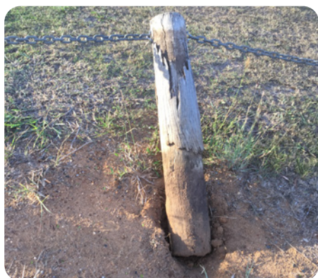
Figure 6.1: Bollards buried in ground should aim for 600 mm deep to avoid overturning.
