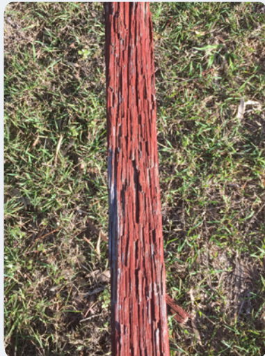
A: Top rail weathering – Some degradation apparent in more than 30 years of weathering.
