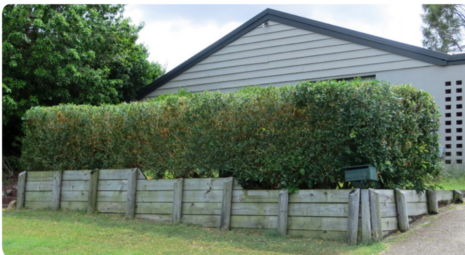
Figure 3.4: Well designed and constructed treated pine retaining wall. Wall is battered and tops of posts have angle cut to shed water
