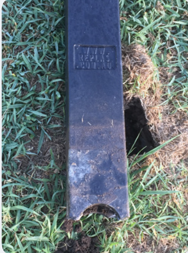
A: Sheared bollard – This new recycled plastic bollard was sheared at the ground by vehicle impact.
