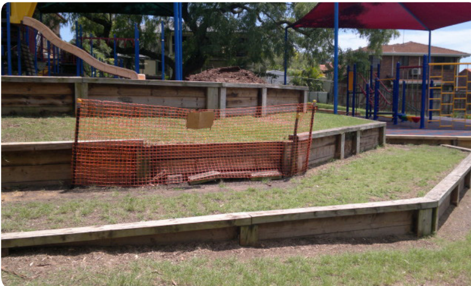
Figure 2.7: Premature failure of incorrectly treated pine sleeper wall in school playground
