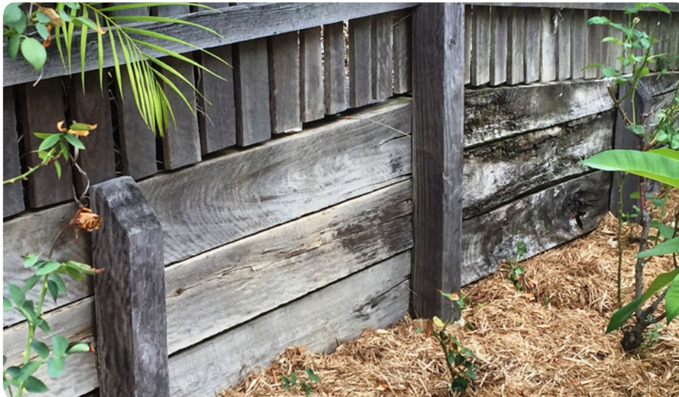
Figure 3.3: Sloping cut to top of ironbark retaining wall post in this 23 year old wall
