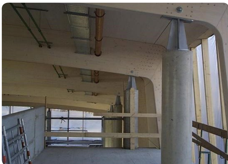
Figure 52: Example of utilities running through high strength fibre reinforced glulam beams instead of underneath such as required in unreinforced glulam
