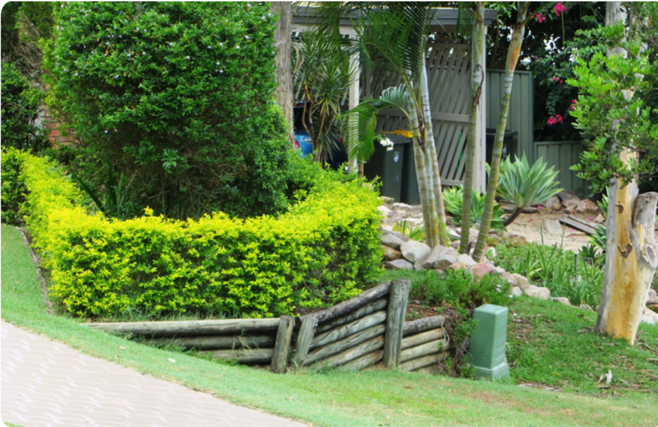
Figure 1.2: It is critical that the footing embedment of posts is adequate to prevent rotation of the posts. The treated pine rounds in this wall are still sound. The wall is failing due to inadequate embedment of posts.
