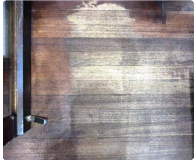
Figure 3.47: Coating degradation due to abrasive wear.
