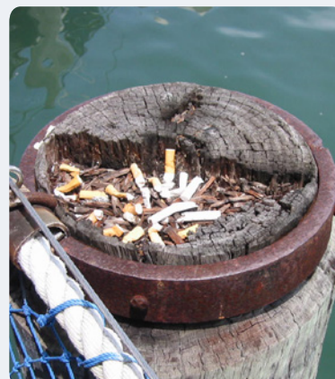
C: Deterioration at heart – Traditional steel banding to bollard ends does nothing to protect the post from weathering.
