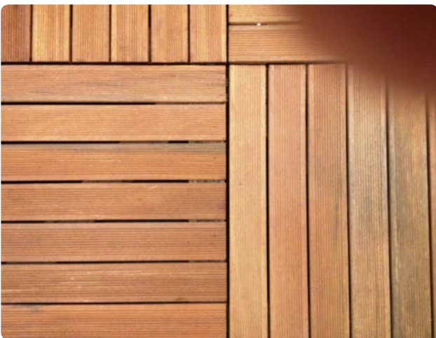
Figure 3.21: Chequerboard configurations can give the illusion of slip resistance.
