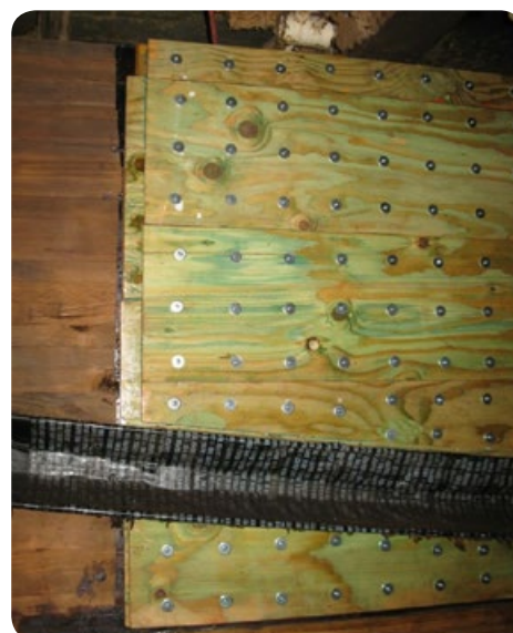
Figure 53: Example illustration of shear panels utilised around services to provide for adequate net shear resistance in the glulam element
