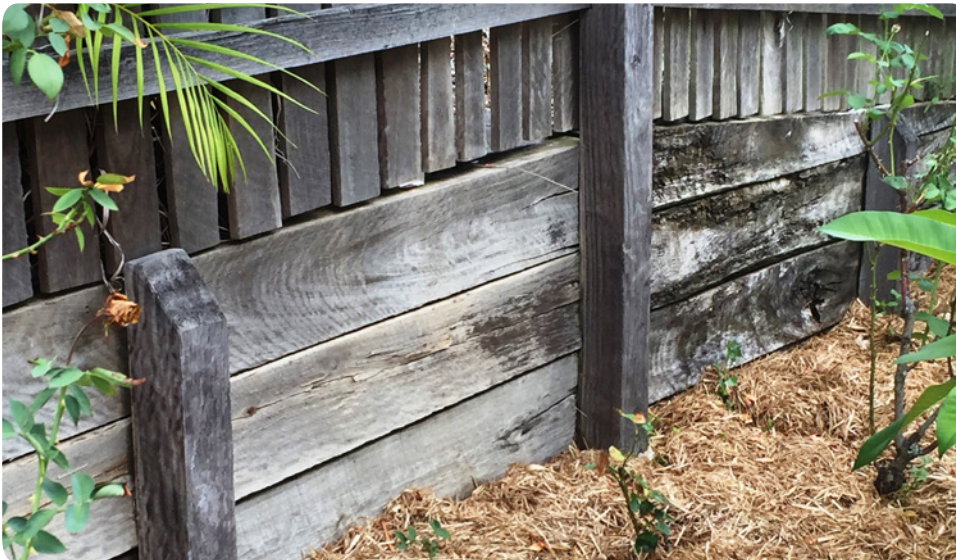
Figure 3.3: Sloping cut to top of ironbark retaining wall post in this 23 year old wall
