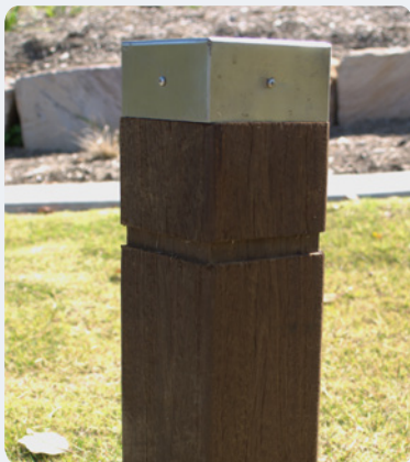
A: Over-fitted – Simple push-on end cap requires accurate symmetrical post cutting and ideally discrete fixing.
