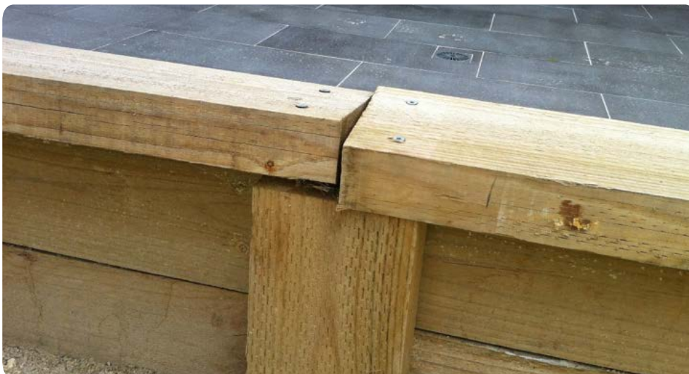
Figure 3.7: Inadequately fixed (screws of insufficient length) resulting in distortion (twisting) of sleepers used on flat.
