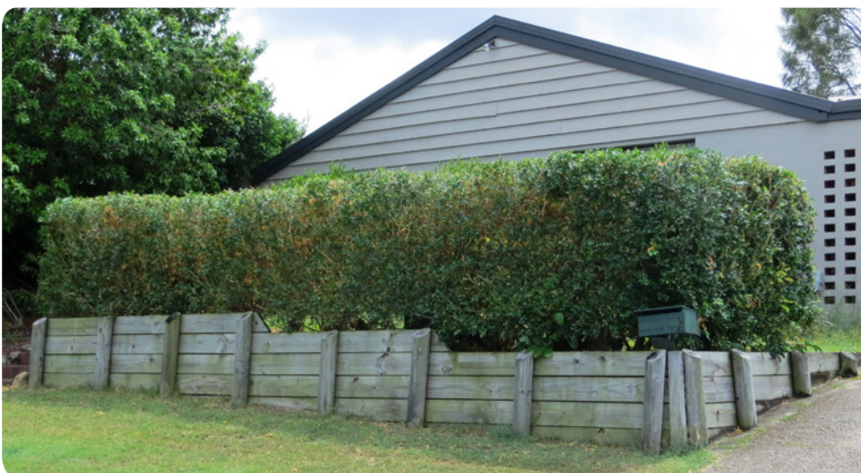
Figure 3.4: Well designed and constructed treated pine retaining wall. Wall is battered and tops of posts have angle cut to shed water
